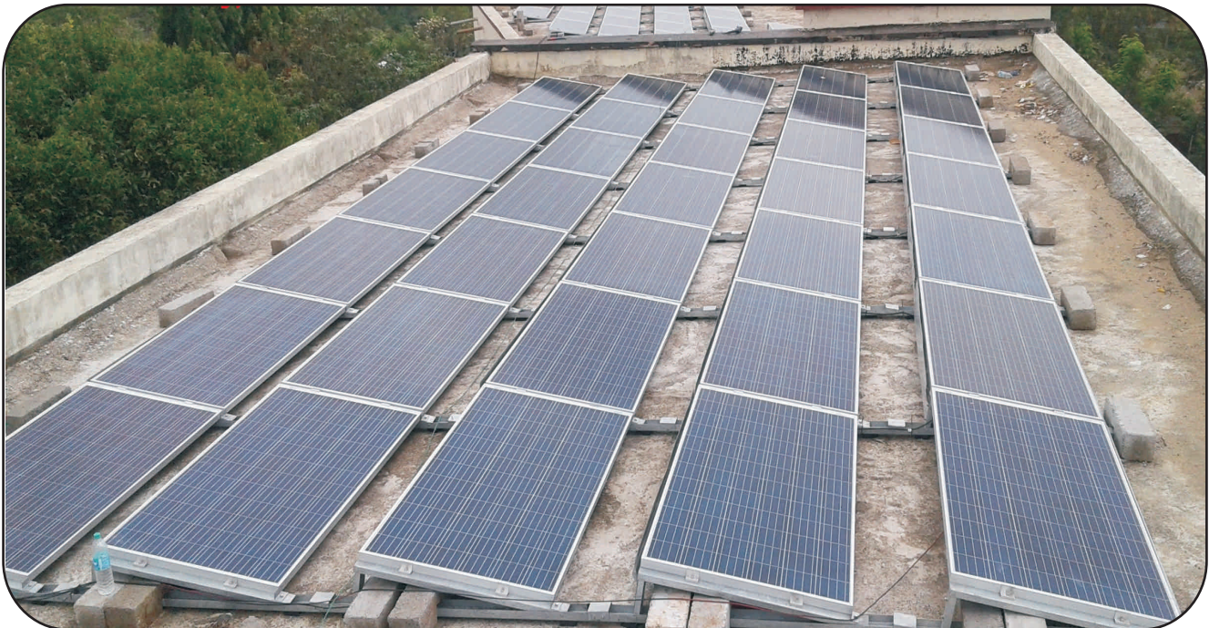
223.82 KWP Rooftop Solar Installed at Utkal University, Bhubaneswar
