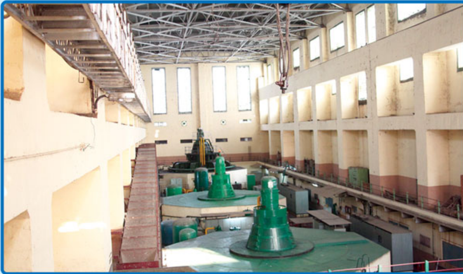
Machine Floor, CHEP, Chiplima
