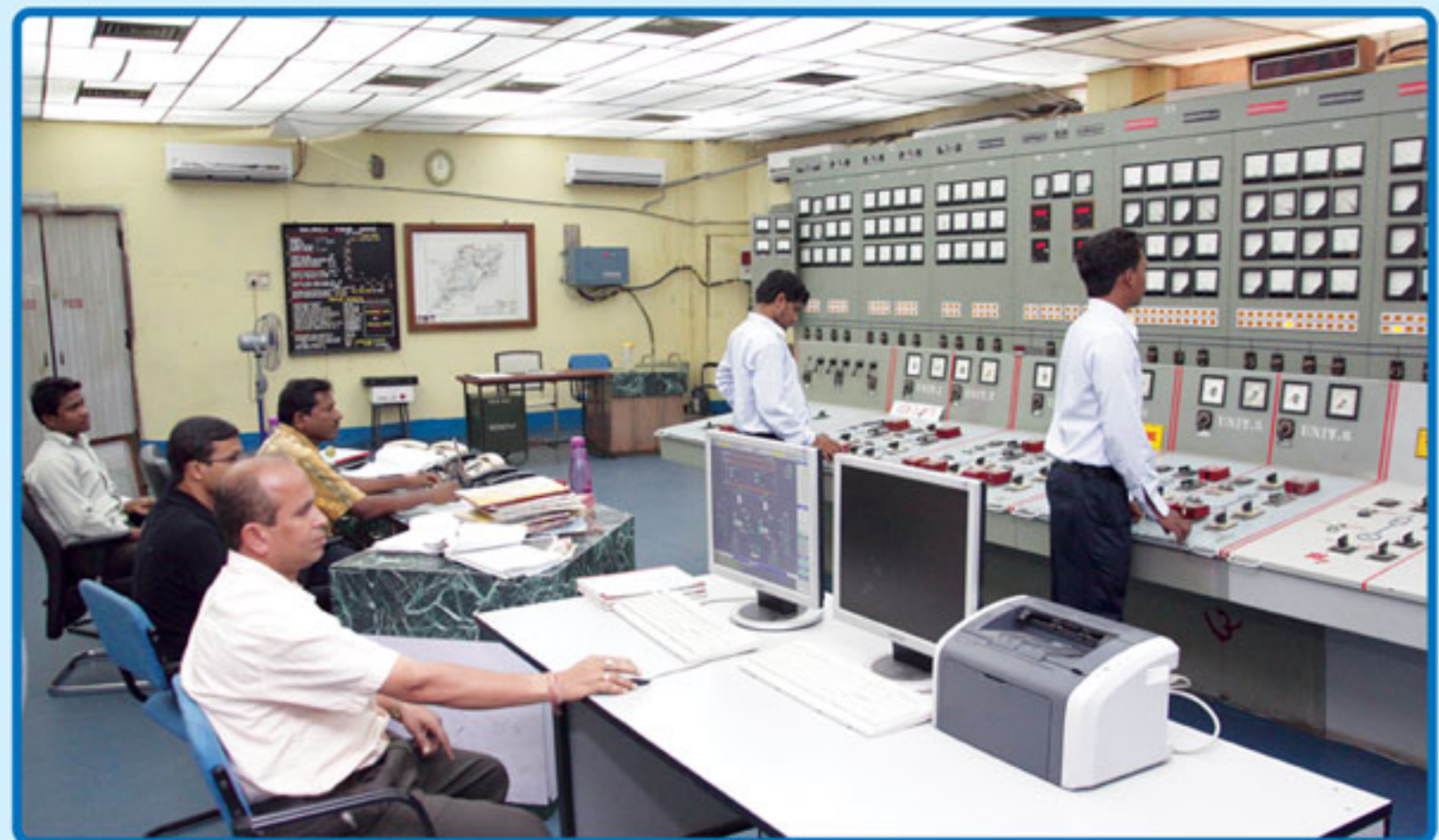
Main Control Room of BHEP, Balimela
